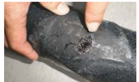
➤ Cable faults on paper-insulated mass-impregnated cable
